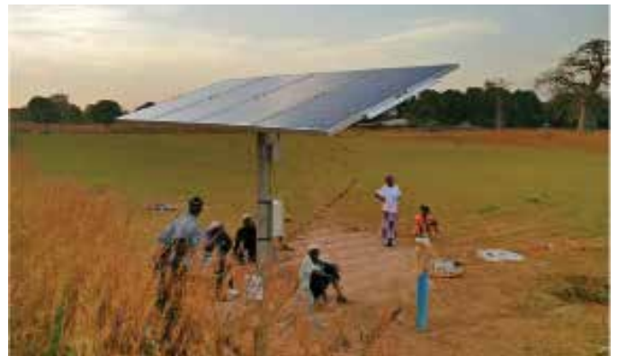
The solar panel that powers Sintet's water pump © Project Gambia
